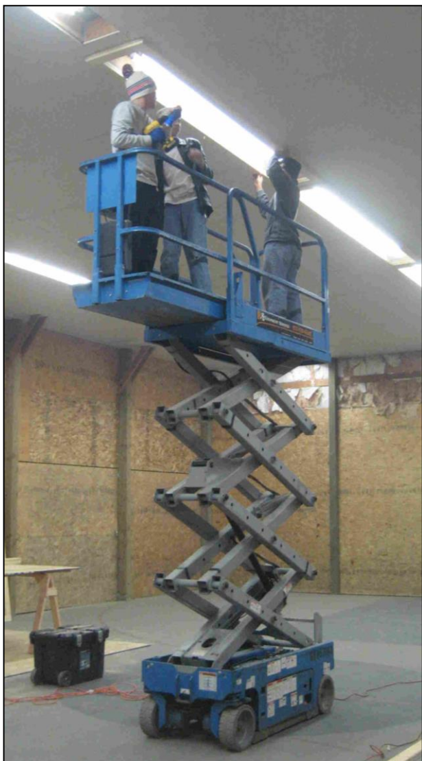
The seminarians use our new lift to install covers over the gym lights.
