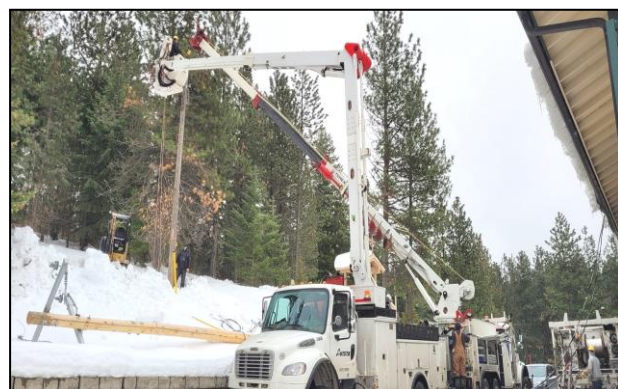
Despite the snow, the local power company replaced our aging power pole that supplies electricity to the seminary.
