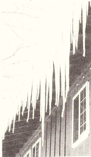
The icicles hanging by the laundry room windows are over six feet in length.
