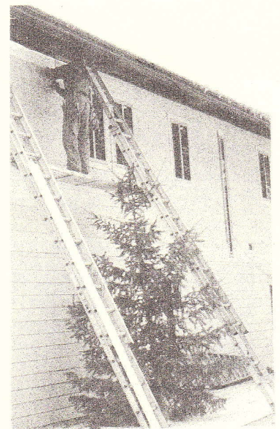
Parish workers continue installing new siding on our seminary, even in the cold weather.
