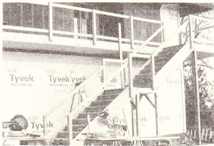
The seminary gets a new deck and outdoor entrance on the east side of the building.
