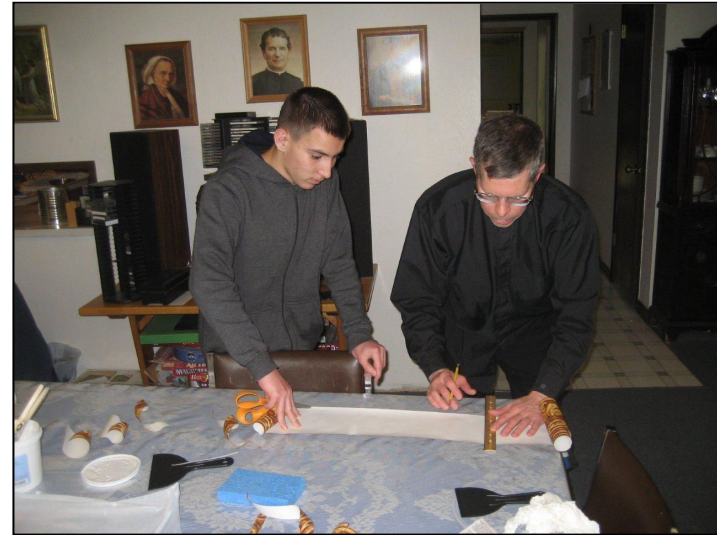
Robert was a big help in measuring, cutting, gluing and installing the wallpaper.
