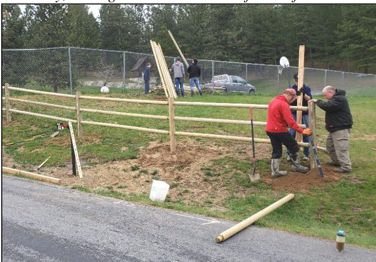
On a recent Saturday the seminarians learned how to install a split rail fence for our church property.
