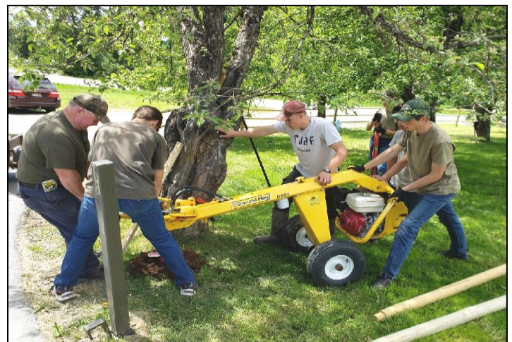
Mr. LeStage supervised the seminarians in digging holes for the posts for our new fence.
