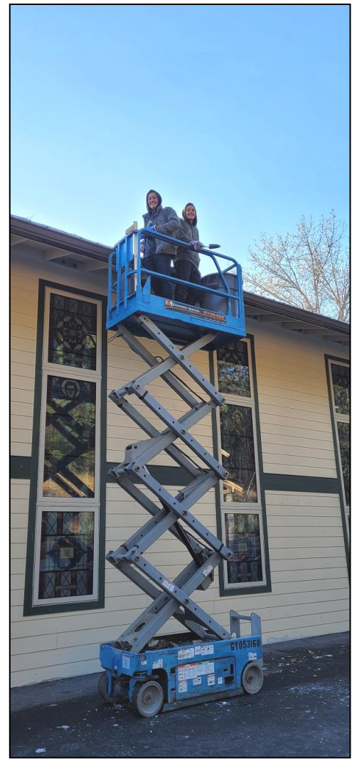
An important fall job is cleaning the leaves out of the gutter along the north side of the seminary.
