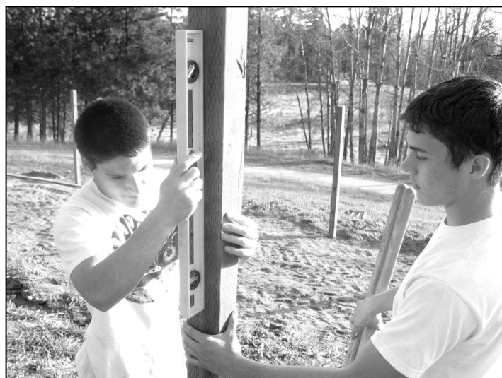
Robert holds the post steady as Zachary uses a level to make sure it is straight.
