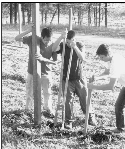
We spent most of a Saturday digging holes and placing the fence posts.
