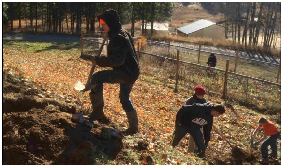
One recent project was the digging of a trench for a propane line to the seminary.
