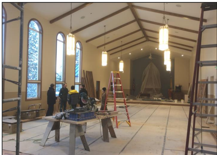
The seminarians take a few minutes to inspect the progress of work on our church.
