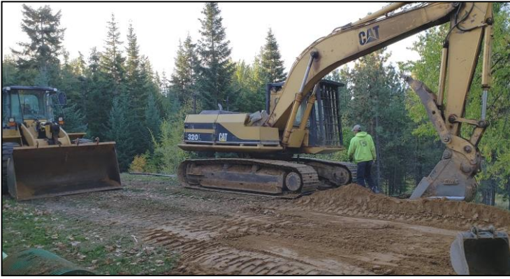
The workers used heavy equipment for the various projects at the City of Mary.
